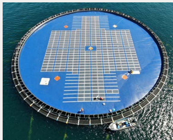
Floating solar system, Statkraft plant in Albania. R&D project. Concept developed by Norwegian company Ocean Sun. This solution requires little material per kilowatt. Each unit basically consists of only a membrane, plastic floating rings and anchoring equipment, and the solar panels.
